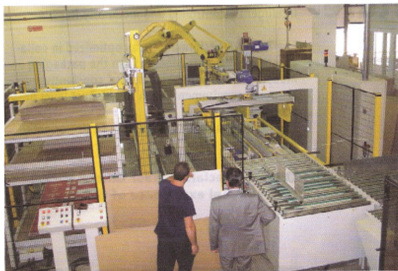
The NE Engineering robotic palletiser behind the EMBA casemaker in the corrugated box plant.
